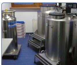
Containers for liquid nitrogen
